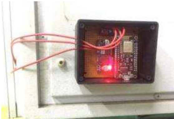
Gambar 4. Hardware transmitter mesin
